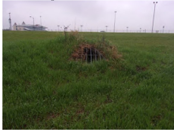
24" RCP directing water to area A
