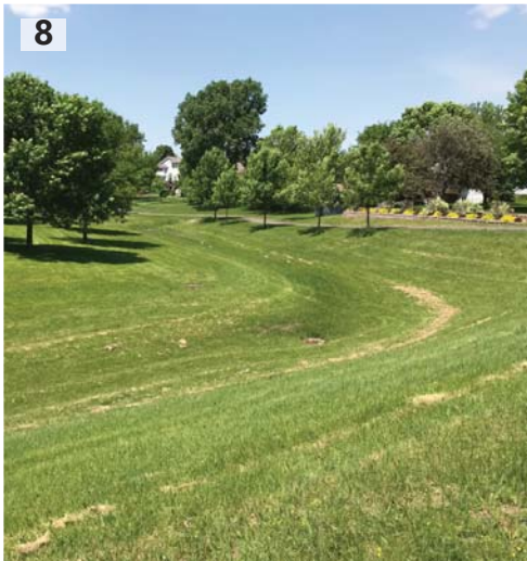
8 OVERFLOW DRAINAGE SWALES ARE HEAVILY MANICURED, NOT PROVIDING NATURAL MEANS OF SLOWING AND FILTERING WATER.
