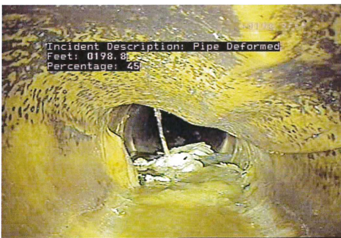
D - Pipe Deformed @ 198.8 ft.
